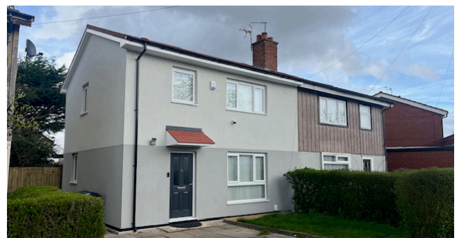
A good example of fault free retrofit installation we have managed
