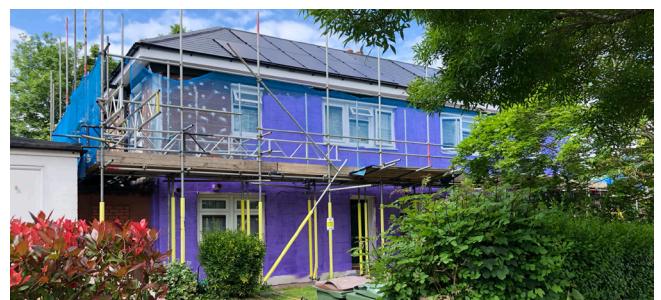
A good example of fault free retrofit installation we have managed
